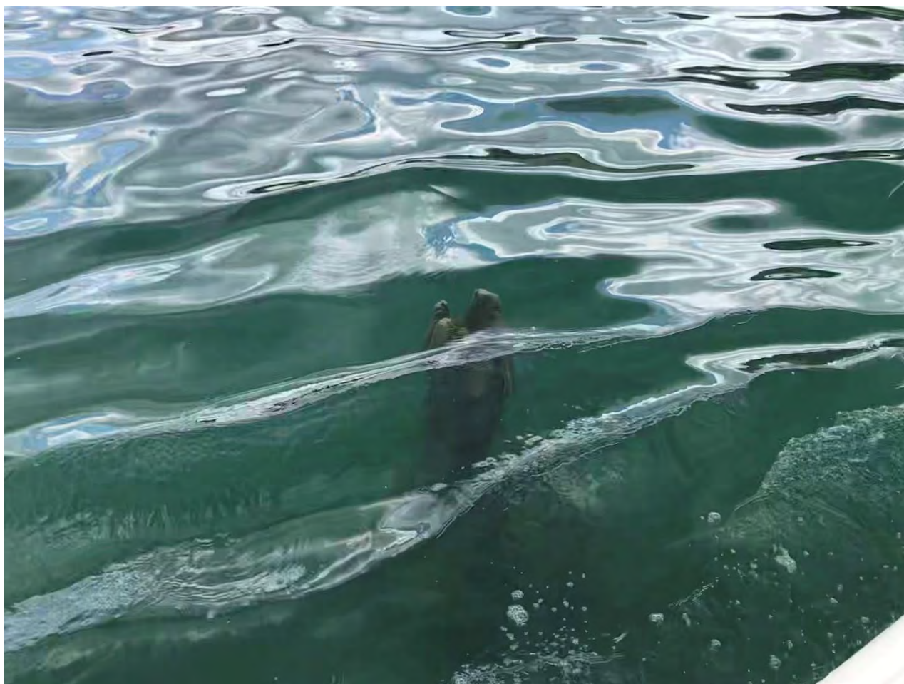
Figure 6: Pier piling at Dean's Pier/Carlton, just below the water's surface.
