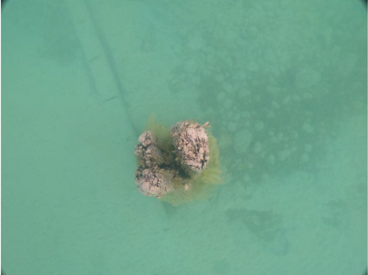
Figure 62: Structural timbers at the base of a standing piling (upper left). Photo taken looking down from just below the water's surface.
